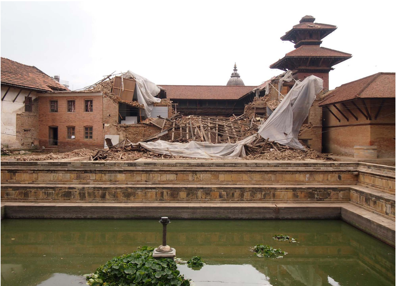
The collapsed East wing of Sundari Chowk Palace | April 25, 2015 The East wing which was built in 1936 was the only palace structure that collapsed. All other and recently restored palace buildings survived the earthquake.
