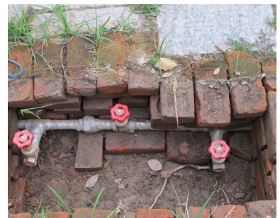
Main water line to Tusha Hiti step well This is the location of a future man hole where water will be diverted to a filtration system.
