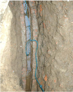
Historic water supply The terra cotta channels dating from the 17th century were restored
